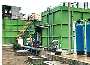
ASP (Activated Sludge Process)
