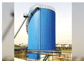
UASB (Upflow Anaerobic Sludge Blanket Reactor)
