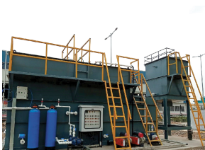
MBBR (Moving Bed Biofilm Reactor)
