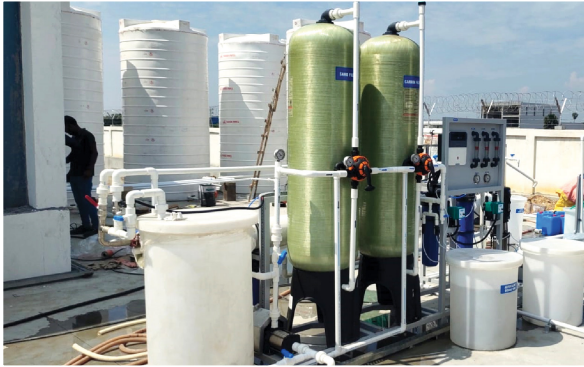
Indospace, Pune (WTP)
